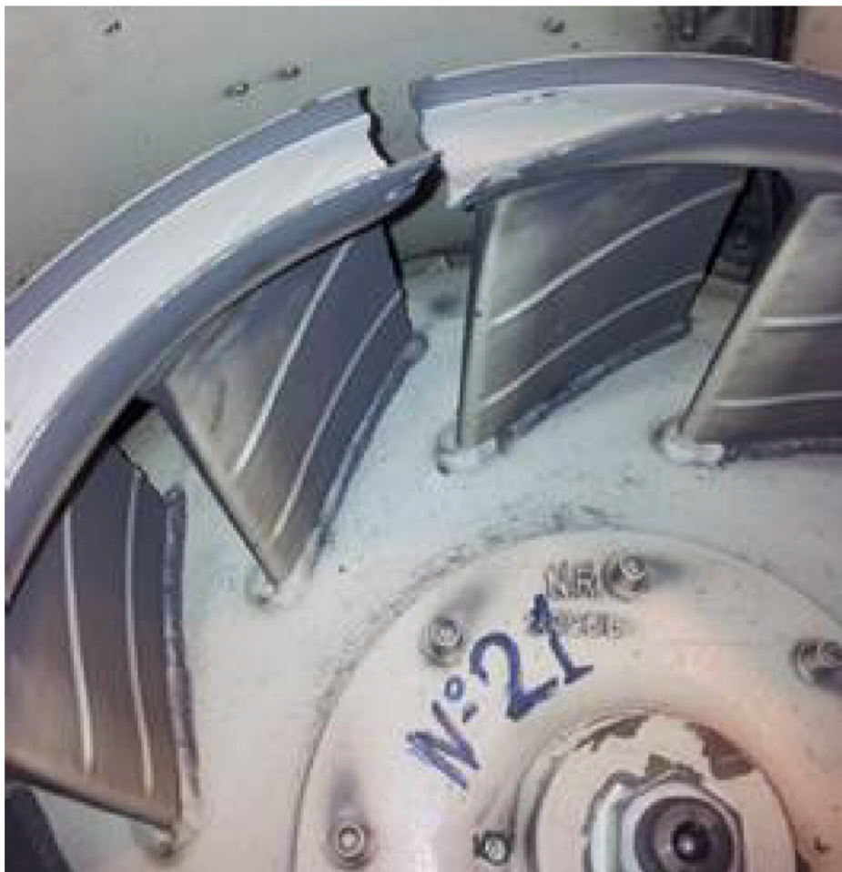
Figure 5. Service-affecting failure of a traction-motor blower. Note how the turbine has been heavily deformed before breaking.
