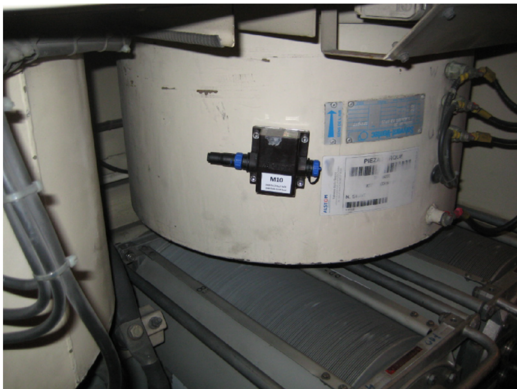
Figure 2. TheMotes installed on the outer casing of the traction-motor blower.
